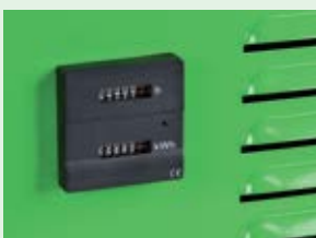
Power meter, installed
